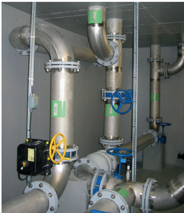
Figur 7.1: Ventilkammer under basseng
