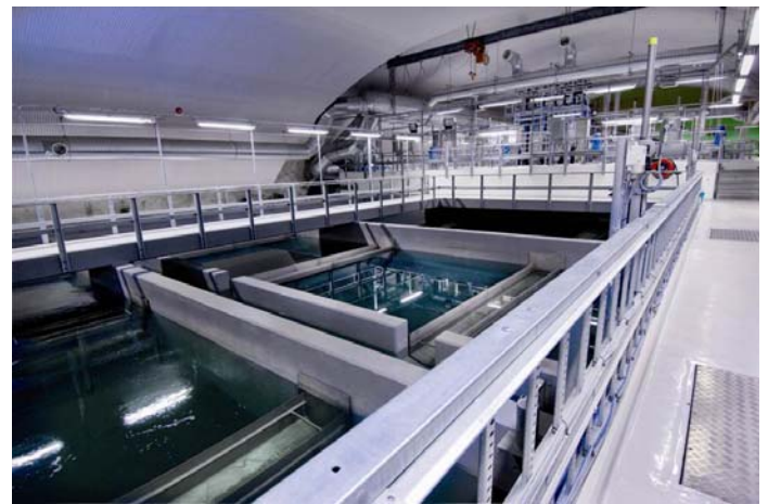
Sand filtration basin
